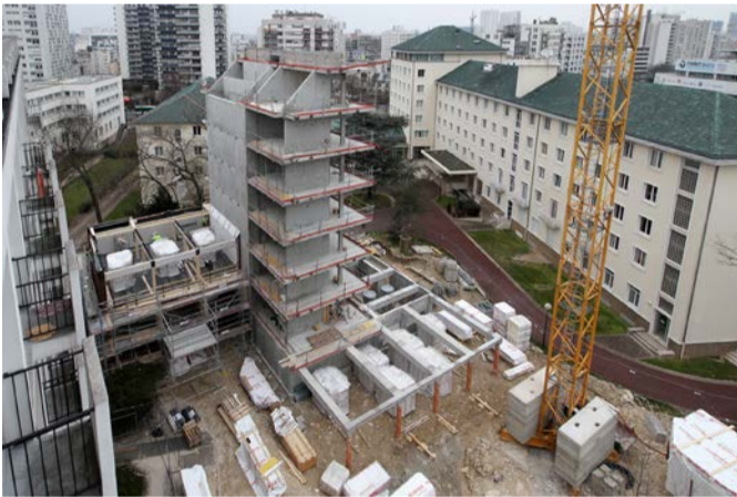
The concrete core is completed, the installation of the wooden structure starts for the western part of the project.
